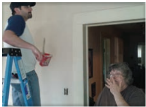
Susan B. looks on with delight as volunteers make much needed repairs to her home.
